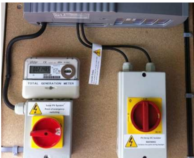
Figure 95: Overcurrent protection devices (OCPDs)
