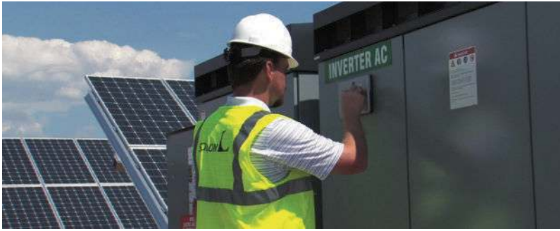
Figure 78: Note readings from inverter display screen
