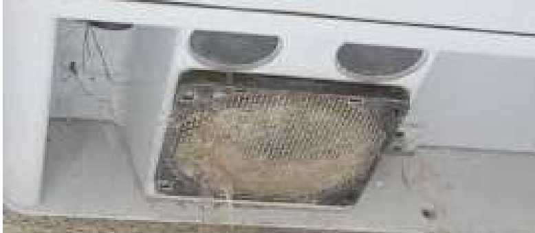
Figure 88: Dust accumulation on Inverter
