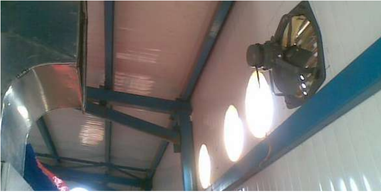
Figure 87: Inverter ventilation room
