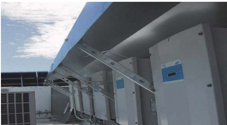
Figure 85: Inverter installed under shade
