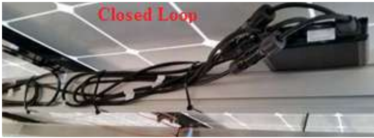
Figure 102: Incorrect cables connection looped tightly
