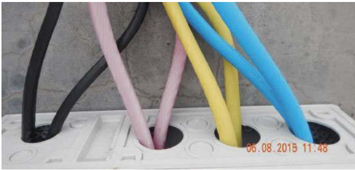
Figure 107: Incorrect – Cable conduit are not closed
