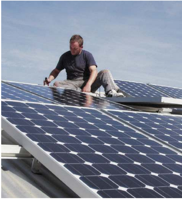
Figure 160: Incorrect practice - Without safety belts
