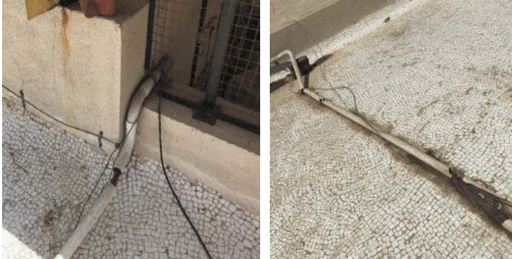
Figure 109: Incorrect - Conduits are damaged
