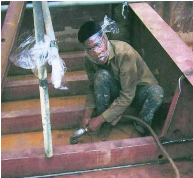
Figure 154: Incorrect practice - Without face shield
