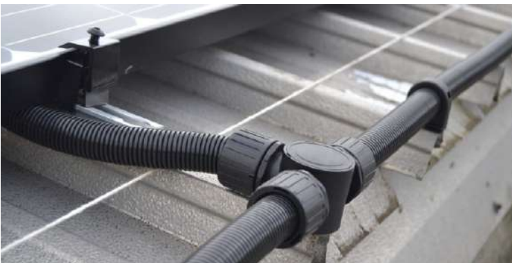
Figure 110: Correct - Conduits are in proper condition
