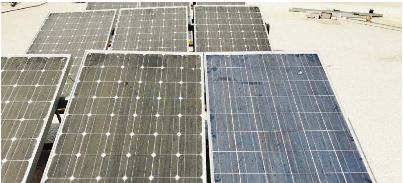
Figure 31: Two modules – one of mono-crystalline and the other polycrystalline technology installed in the same system
