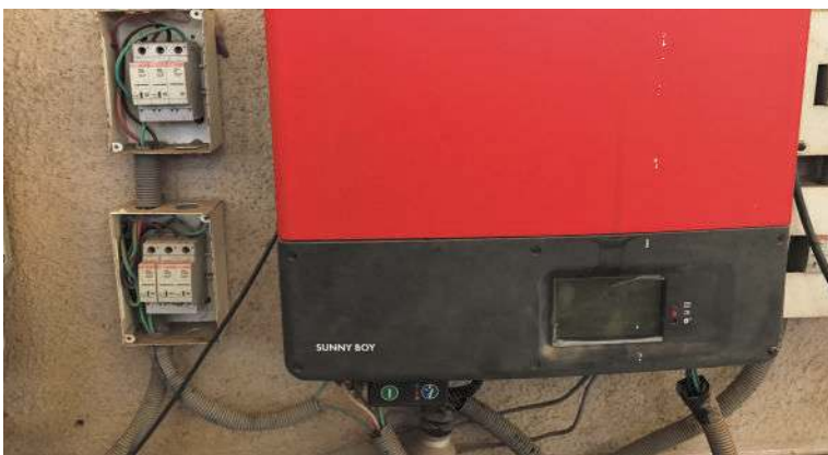
Figure 86: Inverter cables and conduits got loose
