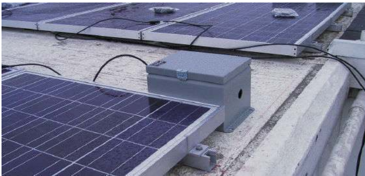
Figure 100: Incorrect cable routing
