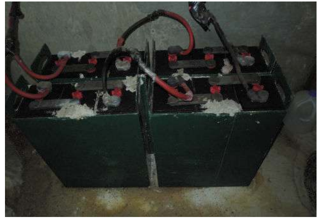
Figure 127: Improper condition of battery
