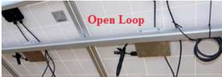
Figure 103: Incorrect cables connection looped loosely
