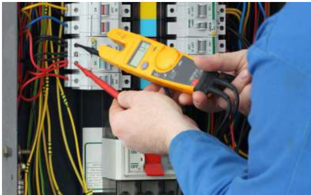
Figure 158: Incorrect practice - Without safety gloves
