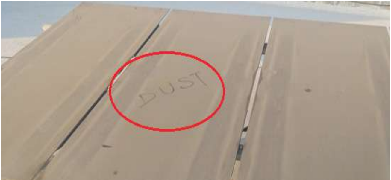
Figure 25: Cleaning required (Significant financial impact)
