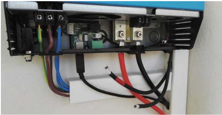
Figure 83: Disconnected wire from inverter base
