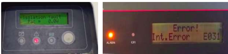
Figure 80: LED Red - Indicating incorrect operation of inverter
