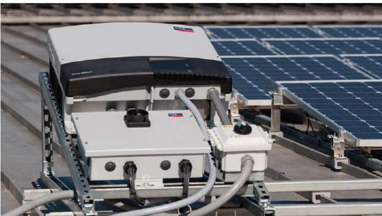
Figure 84: Inverter installed without any shade or roof
